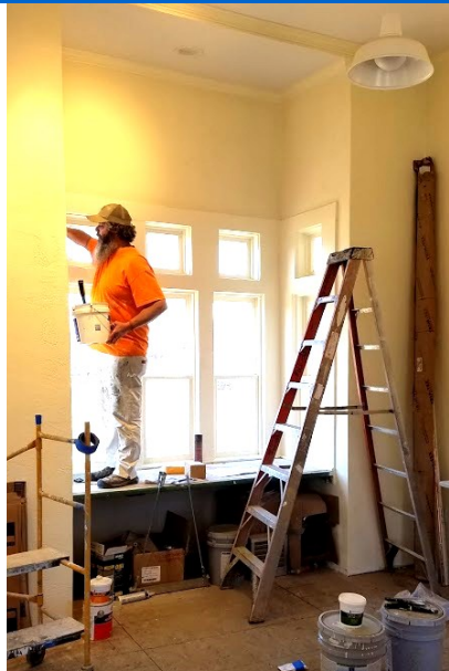
A contractor works on interior painting in the Nickel Plate Station. (Reinhardt)
